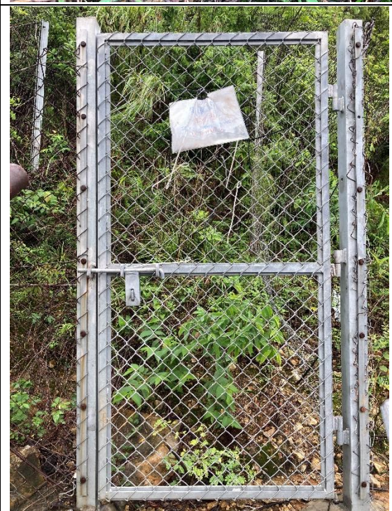
Photo 2 – Current situation of fencing and warning sign
